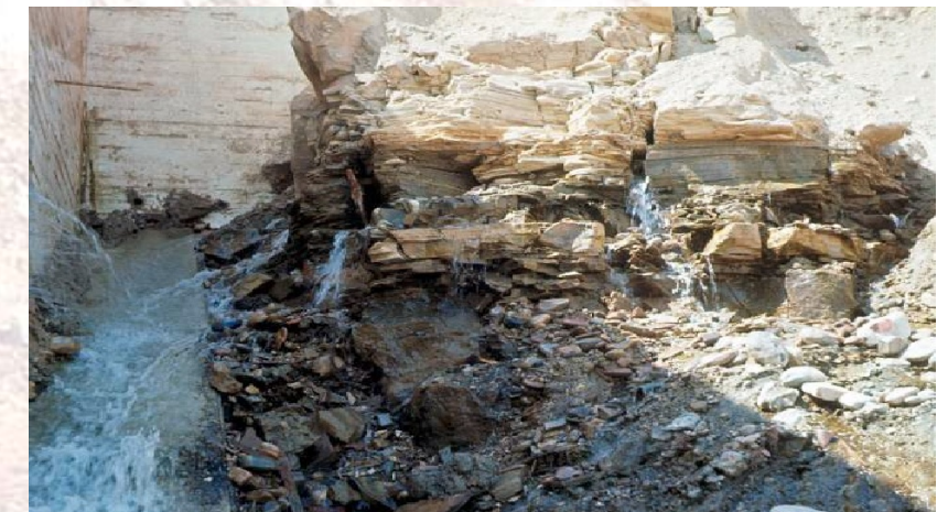
Fontenelle Dam Incident, Wyoming, USA from USBR
