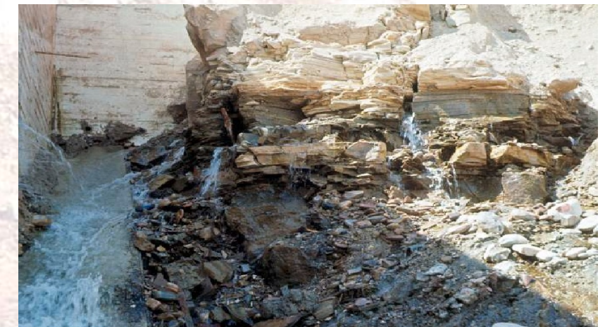
Fontenelle Dam Incident, Wyoming, USA from USBR
